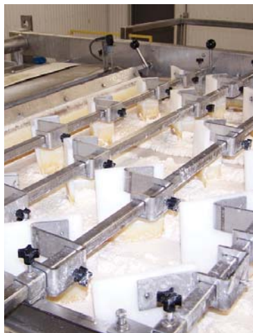
The belt filter press gravity deck in operation.
